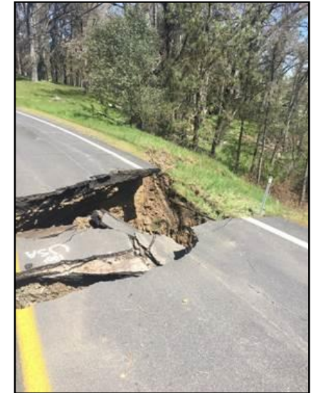
This sinkhole continued to open and became a loss of roadway on 4/15/2018 .
